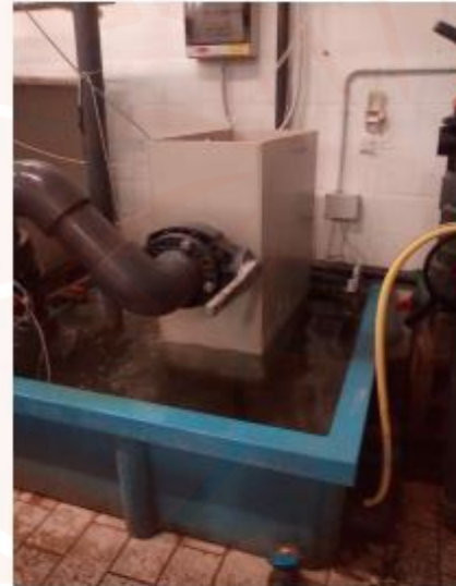
Collection tank with pre-filter
