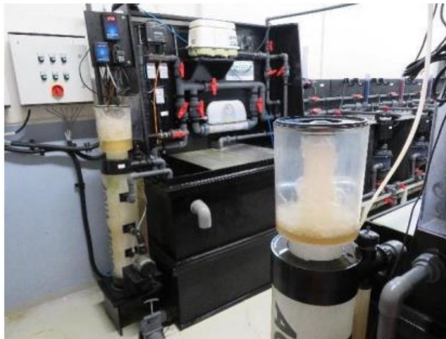
Figure 2: Water treatment system
