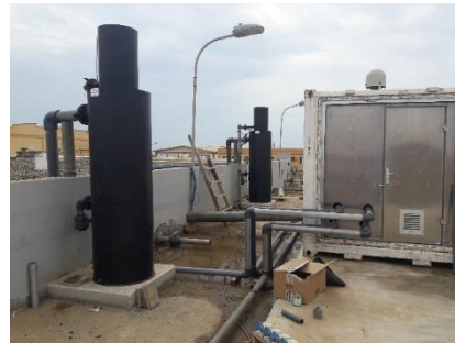
Hatchery containerized set-up
